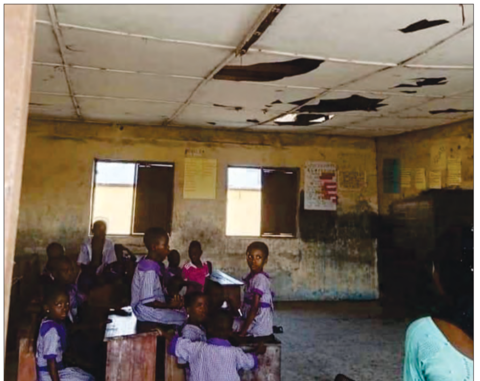
A dilapidated school building in Ibeju Lekki
